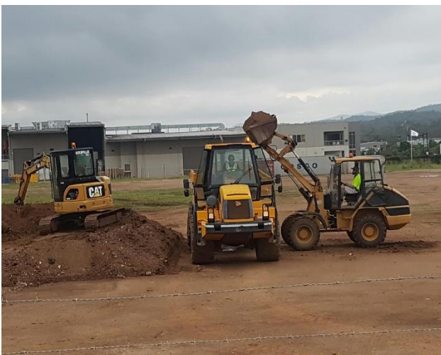
Figure 3 – Students training on plant machines (L-R) Excavator, Articulated Haul Truck & Front-End loader
